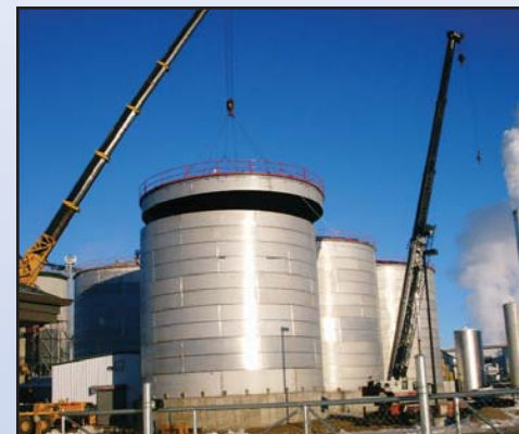
Wimbo, Inc. installs the lid of the additional fermenter which came on line in mid-February. The additional fermenter will increase production.
