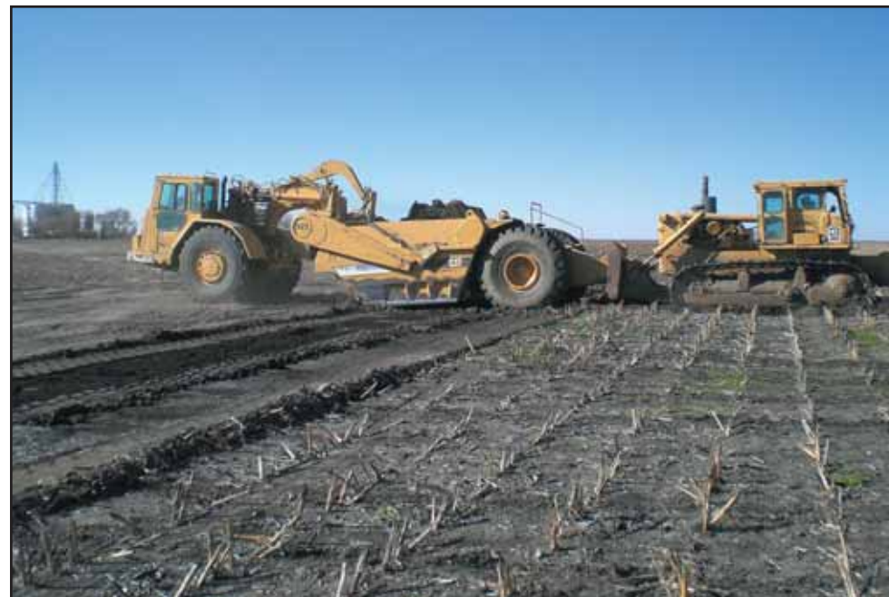
Dirtwork began at Missouri Valley Renewable Energy, LLC near Meckling, SD and Aberdeen Energy, LLC near Mina, SD earlier this month. Pictured is a scraper removing top soil at MVRE.
